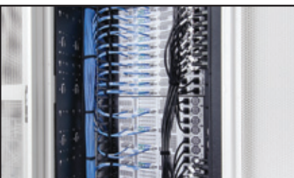
Organized networking and power cable management for proper server airflow
