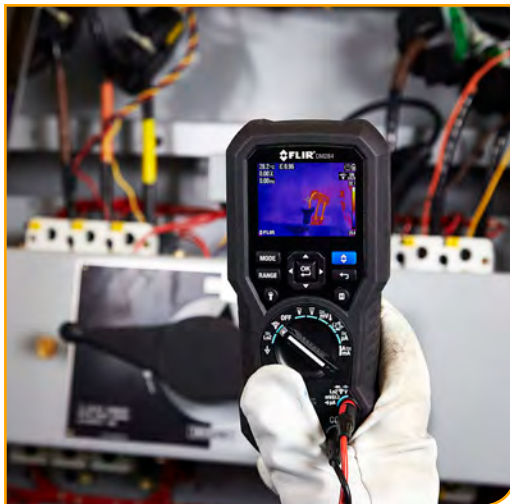
Thermal scan of an electrical panel
